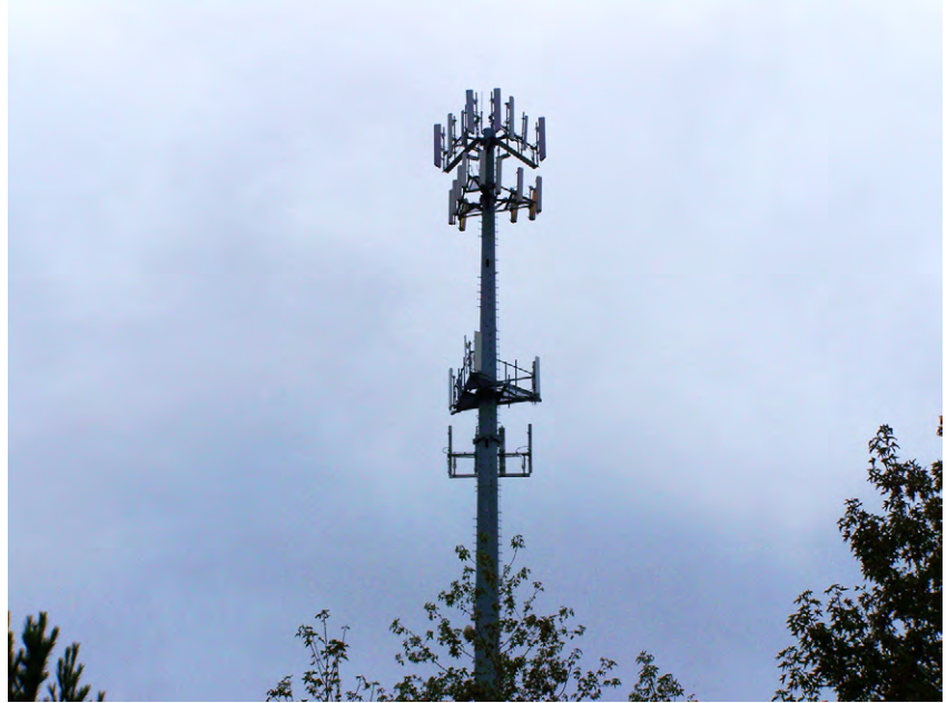
FIGURE 18.1 Cell phone tower
