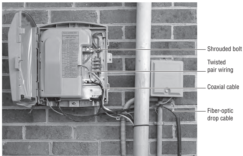
FIGURE 30.11 Network interface device with the cabling entering and exiting from the bottom
